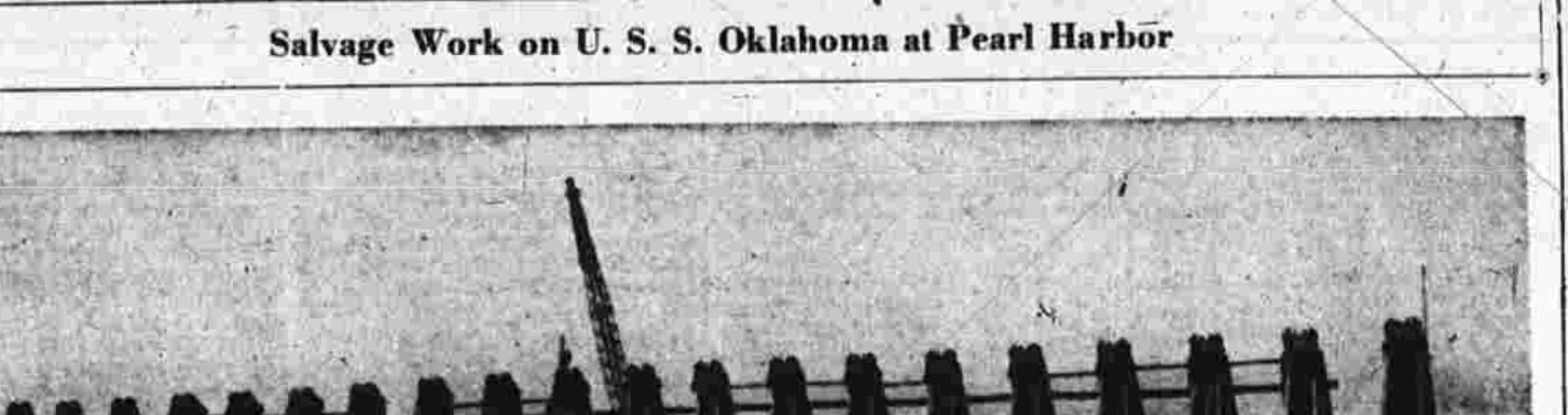
Salvage Work on U. S. S. Oklahoma at Pearl Harbor With the help of huge timber frames, over which run wires attached to winches on the shore, the U. S. battleship Oklahoma, sunk during the Japanese attack on Pearl Harbor, Oct. 7, 1941, is being salvaged.
